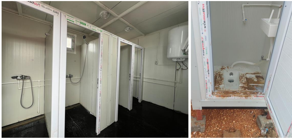
Inaccessible showers and latrines lacking ramp access, handles, ropes or chairs as observed by Amnesty International’s researchers during their March 2023 visit to camps in four of the provinces that were most affected by the earthquakes. None of the 21 displacement sites visited by the researchers contained sanitation facilities that were accessible to persons with disabilities, a wider pattern confirmed by aid workers. © Amnesty International
