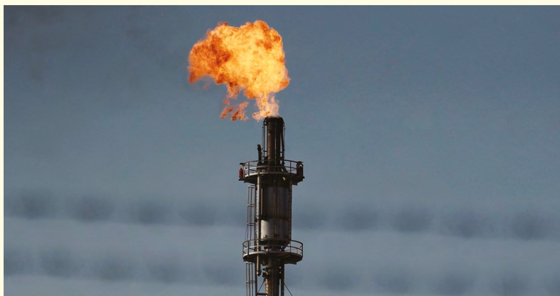
Flames from a flare stack. Flaring is used by petrochemical plants and refineries to burn off excess gas. © 2019 Getty Images/ Bloomberg Creative (Photographer: Dimas Ardian)
