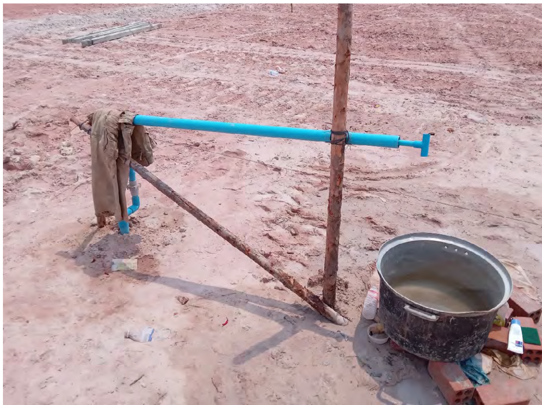
A ground-water pump installed on a land plot at Run Ta Ek resettlement site, July 2023, Amnesty International.
