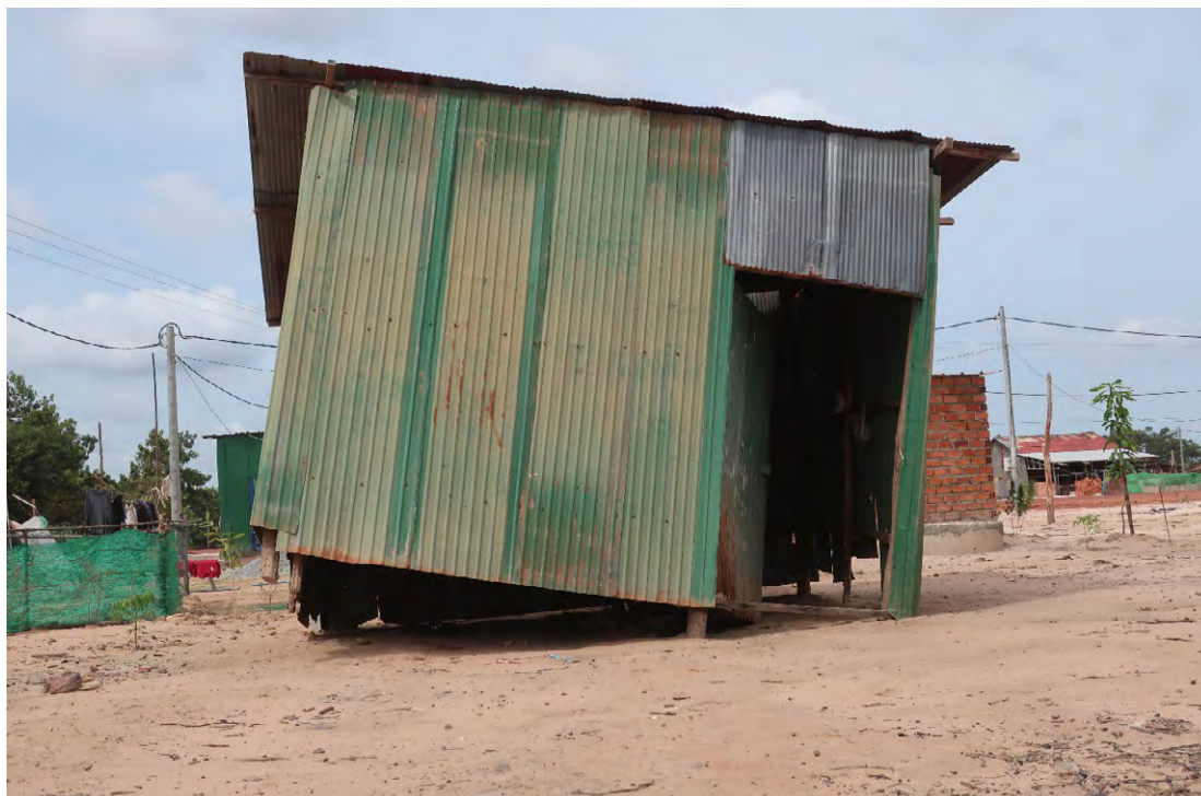
A damaged house at Run Ta Ek resettlement site, July 2023, Amnesty International.
