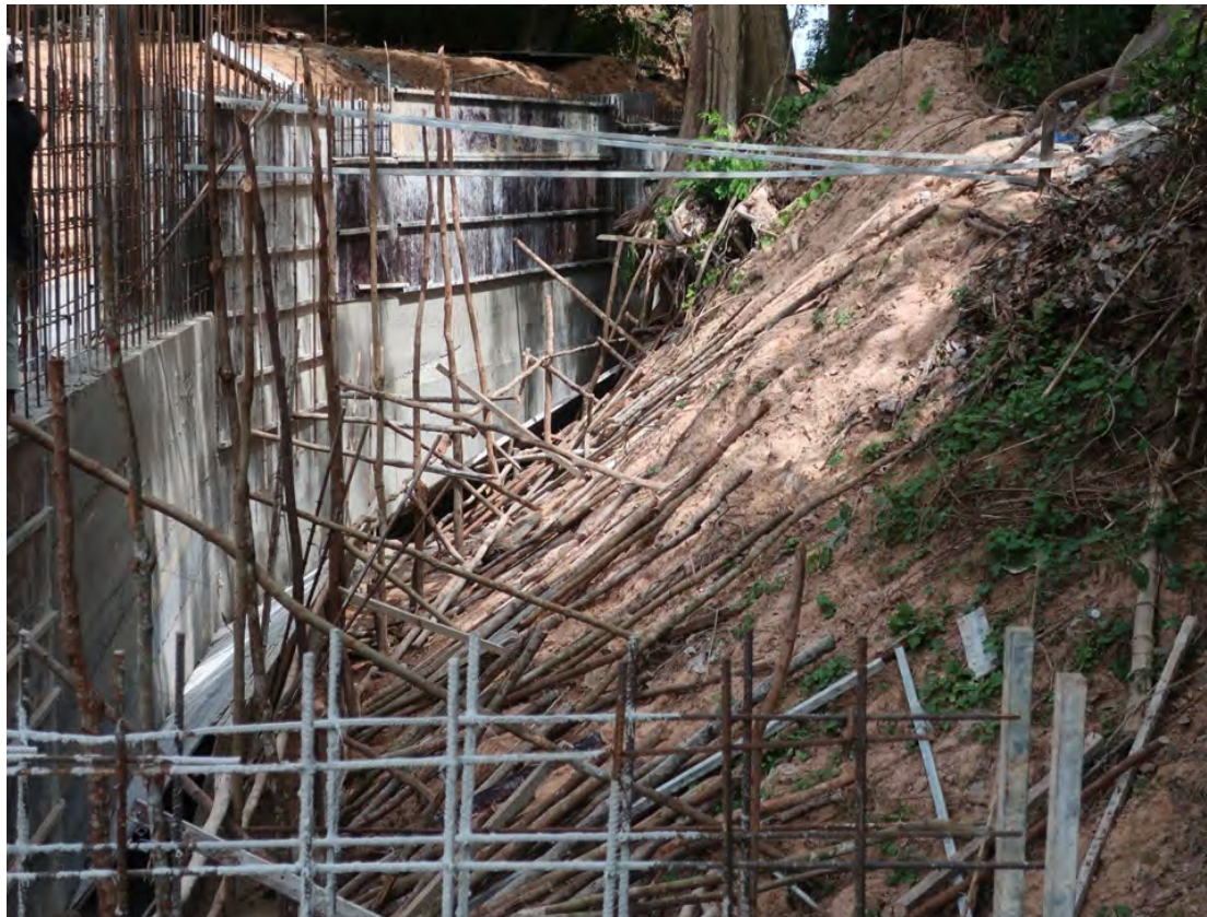
Installation of a dam gate near Rohal that could raise flood levels in Angkor, July 2023, Amnesty International.
