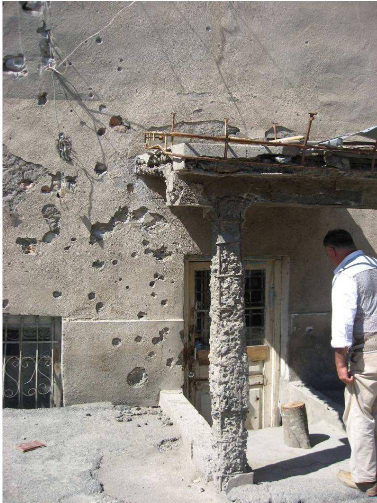
Damaged entrance to a synagogue cellar in Shaumian street, Tskhinvali, where civilians hid during hostilities in August 2008. Tskhinvali, South Ossetia, July 2009. © Amnesty International
